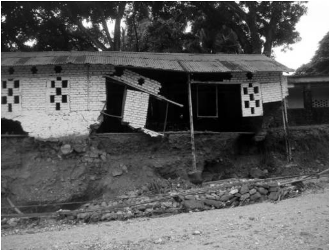
Fig. 2. Destroyed School Building After a September 2009 Flash Flood, Khahare Khola. Photo: Dubois (2009).
